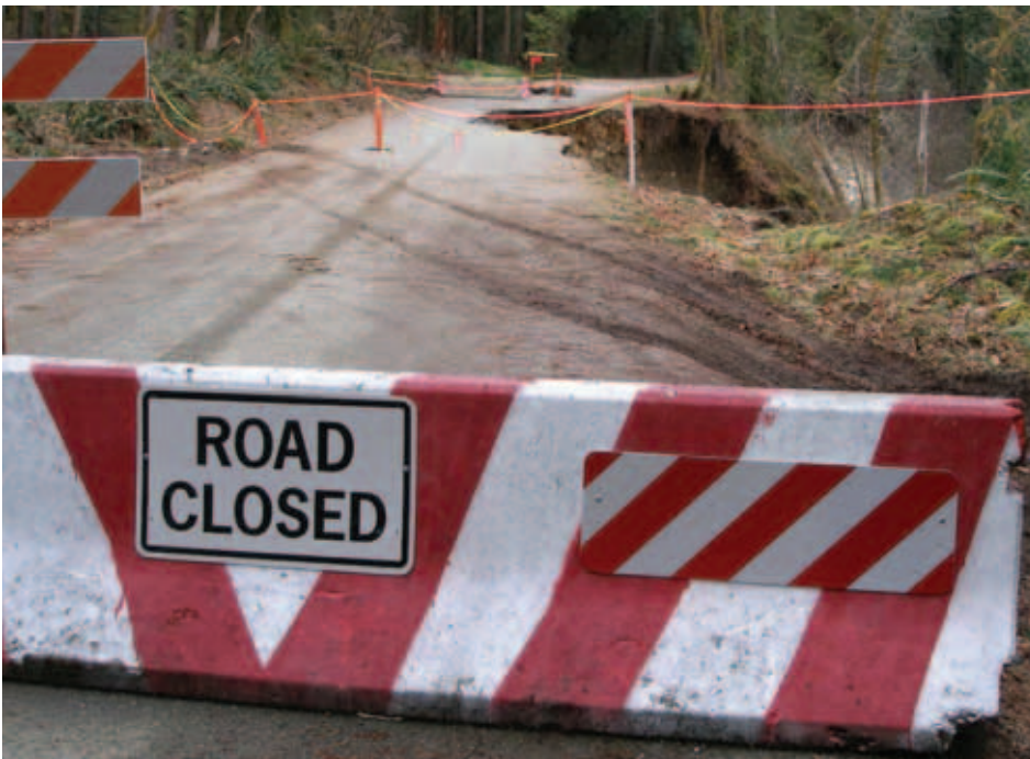
The impassible road 26 above the Suiattle River in the Mount Baker-Snoqualmie National Forest. The river cut into the hillside below the road leading to road failure.
