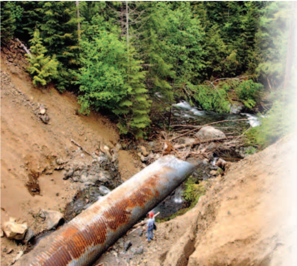
Inadequate funding for maintenance and recent large floods have combined to accelerate damage to both infrastructure and aquatic resources. Here, a failed stream crossing on an unneeded road delivers sediment to a stream on the Olympic National Forest, WA.
