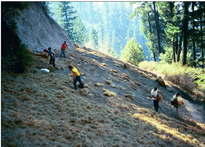
Top Right: Crew on work-site in California restoring roads. Above: Workers revegetating what was once an old road that’s been recontoured. Photos: David Burns
