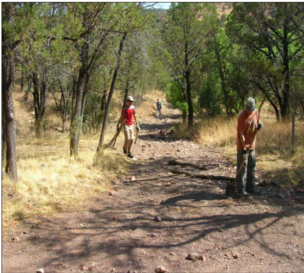
Page 2: Restoration crew improving water quality and fish habitat on the Olympic National Forest in Washington by removing unneeded Forest Service roads. Photo: Steve Zugschwerdt. Above: Restoration work to improve wildlife habitat and prevent soil erosion on the Coronado National Forest in southern Arizona. Photo: Sky Island Alliance Top Right: Montana Conservation Corps revegetating removed road and landing. Photo: Adam Switalski.
